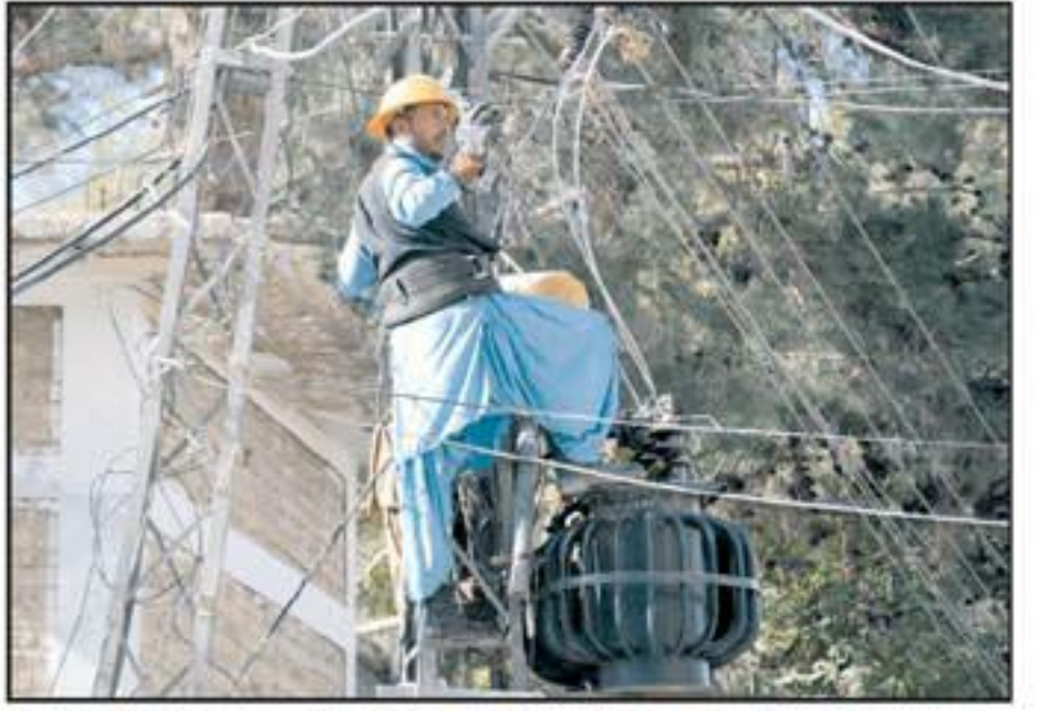
QUETTA: A Quetta Electric Supply Company (QESCO) worker repairing the transformer at Adalat road.
